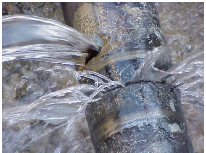
Aging infrastructure like this leaky pipeline contributes to system losses and unrecovered cost for municipalities.
